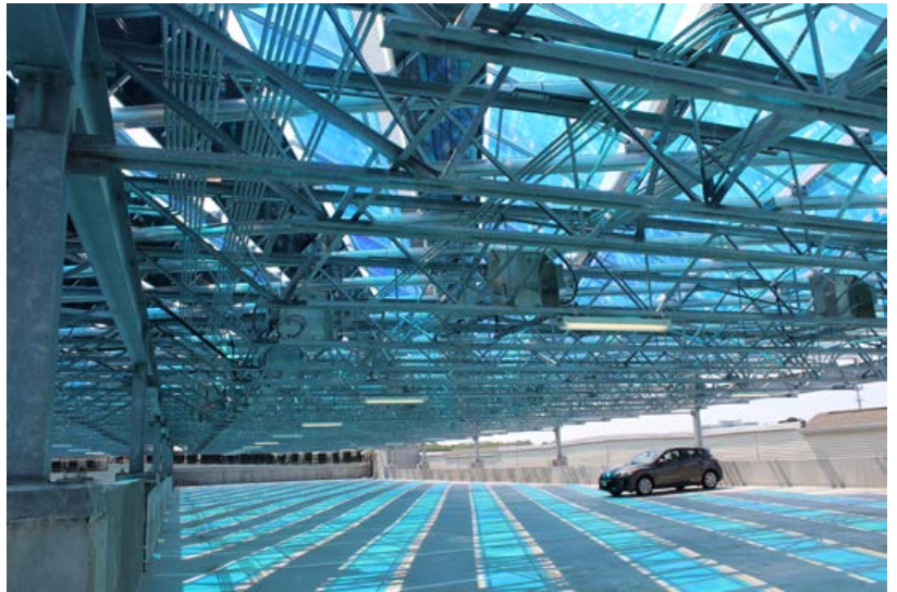
UNDERNEATH THE SOLAR ARRAY
